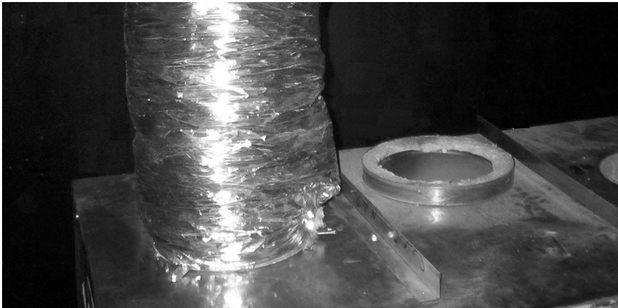
Figure 3 Installation de l'amorce et du tuyau flexible isolé / Gravity vent starter and insulated flexible duct installation
